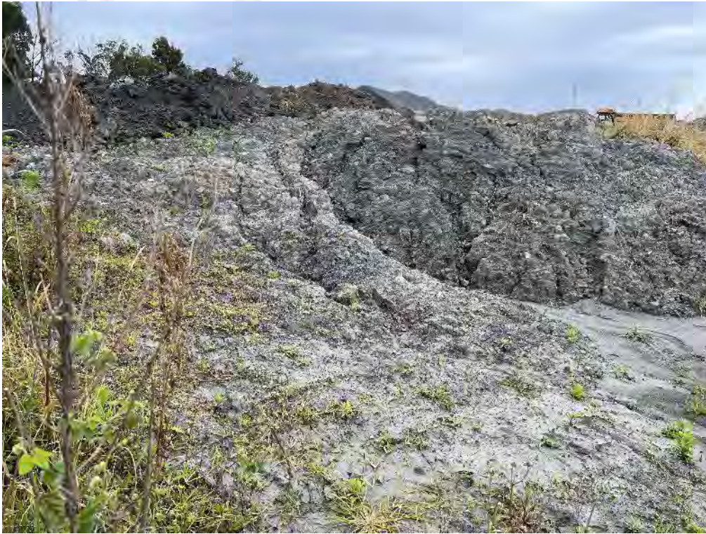
Plate 7: W4 showing erosion of unconsolidated material on the Overburden Stockpile Area – photo from September survey
