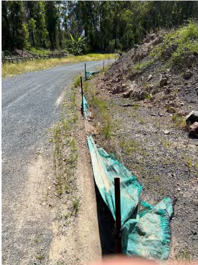
Plate 19: OB12 - Sediment fence in disrepair below topsoil stockpile
