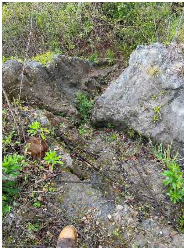
Plate 8: OB1 showing erosion and drainage of material into vegetation adjacent to the Overburden Stockpile Area
